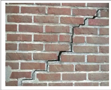
Cracked Brick Can Be a Structural Issue
